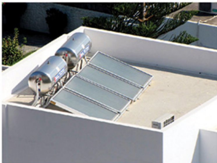
Residence in Skyros island, Solar water heaters with sort height base
