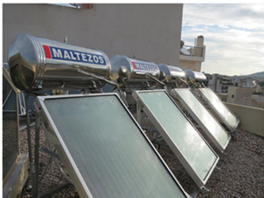
17 Solar water heaters MALTEZOS Inox, Athens, Greece
