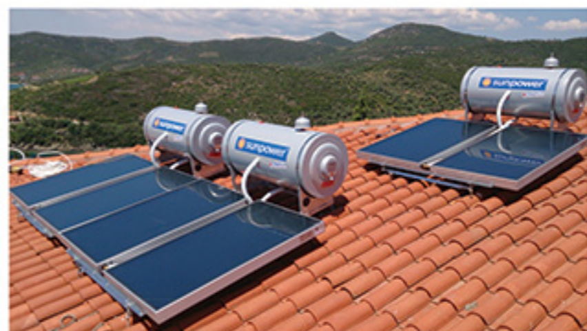
5 Solar water heaters Sunpower, Rooms to rent, Chalkidiki, Greece
