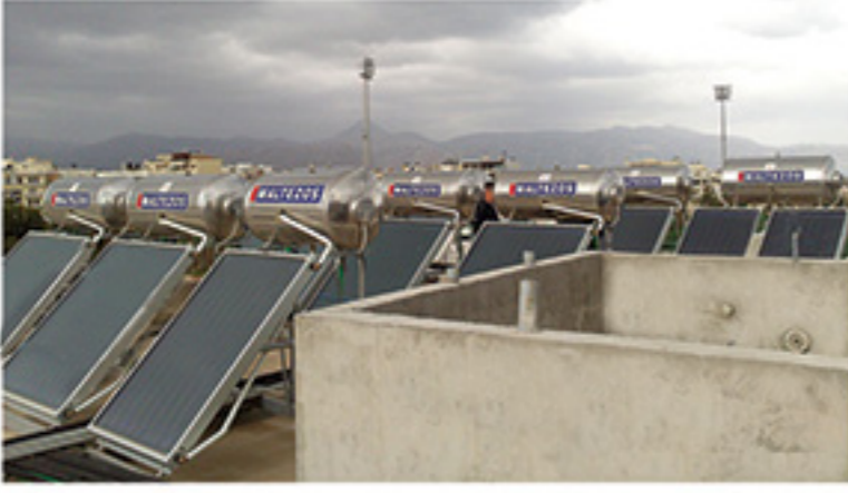
15 Solar water heaters MALTEZOS Inox, Iraklion, Crete
