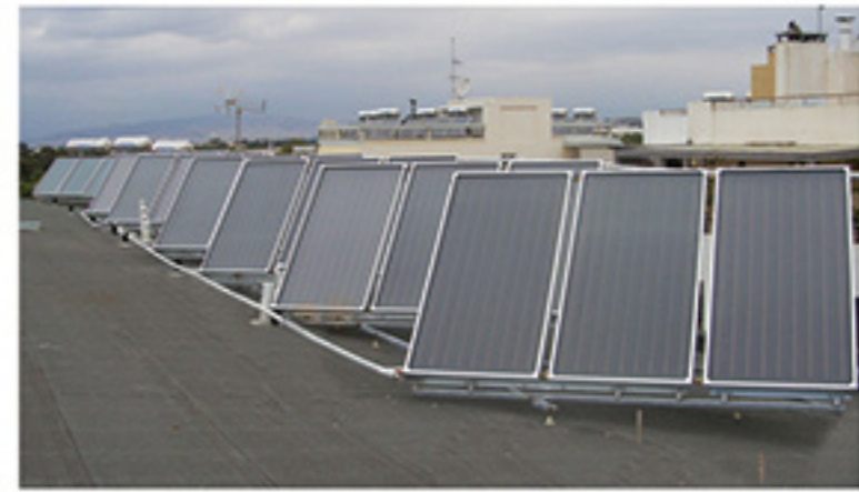
44m 2 selective surface of aluminum collectors, Glyfada, Athens, Greece
