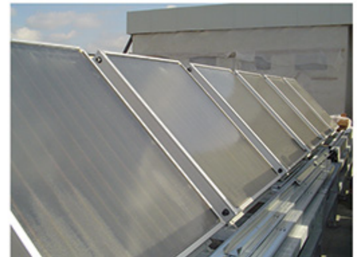
50 m 2 of selective copper collectors, Italia
